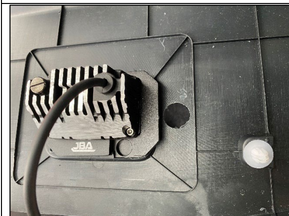
STEP 3.1.3 DRILL THE SWITCH HOLE OUT TO 20MM USING STEP DRILL AS SHOWN. INSERT THE SWITCH AND TIGHTEN NUT FROM BEHIND.
