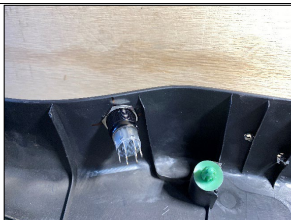
STEP 3.2.5 DRILL THE HOLE OUT 20MM AND INSTALL THE SWITCH WITH NUT FROM REAR AS SHOWN.
