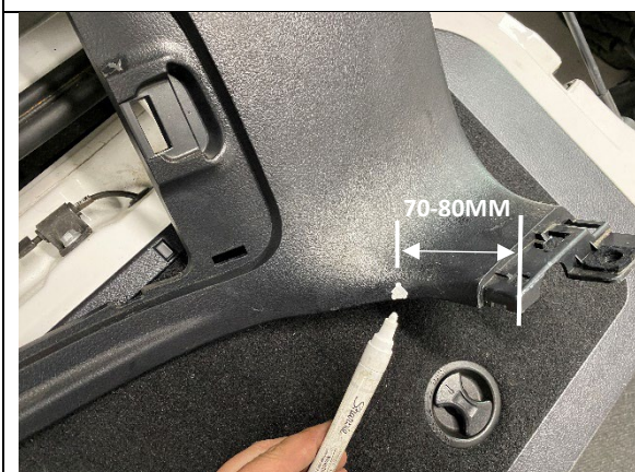
STEP 3.3.3 PREPARATION OF QUARTER PANEL MARK APPROX 70-80MM FROM END AS SHOWN.
